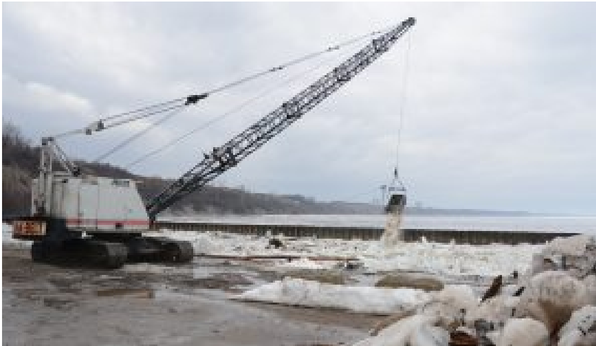
Figure 26: Dragline Crane Removing Ice from Catfish Creek in Port Bruce (Aylmer Express)
