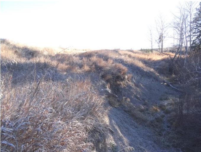
View of sloughing bank (East)
