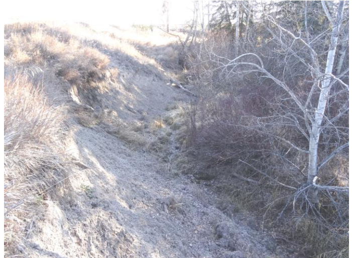
View of eroding bank and stream channel (East)
