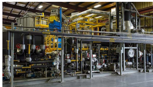
Photo 3: Plastics Pyrolysis Facility
