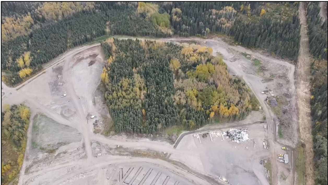
Figure 2. Additional works included contouring the quarry pit for wood waste curing (top left), relocating topsoil piles to one location (bottom left), clearing and developing stockpile area (top right), developing the new public drop-off area (bottom right), construction of 450m of new ditching and installing 4 new culverts.
