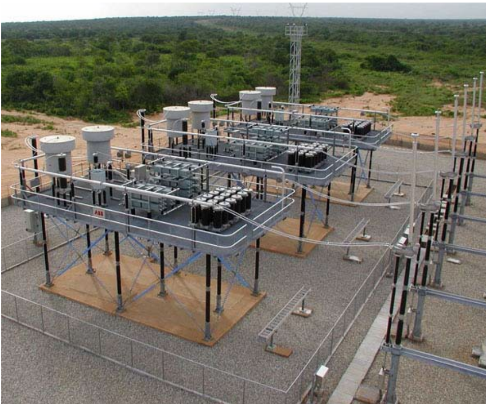
Photo 2 - Typical capacitor bank equipment
