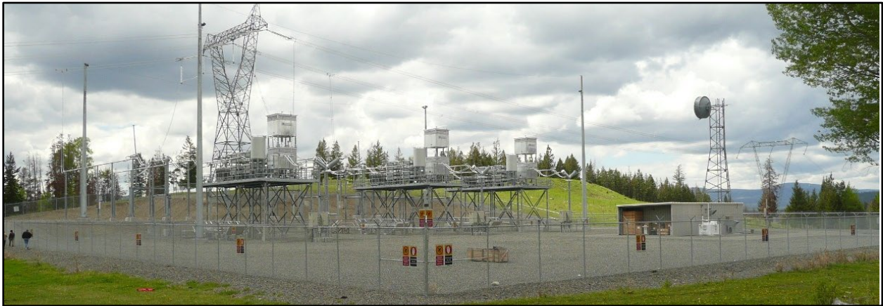
Typical Capacitor Station – BC Hydro
