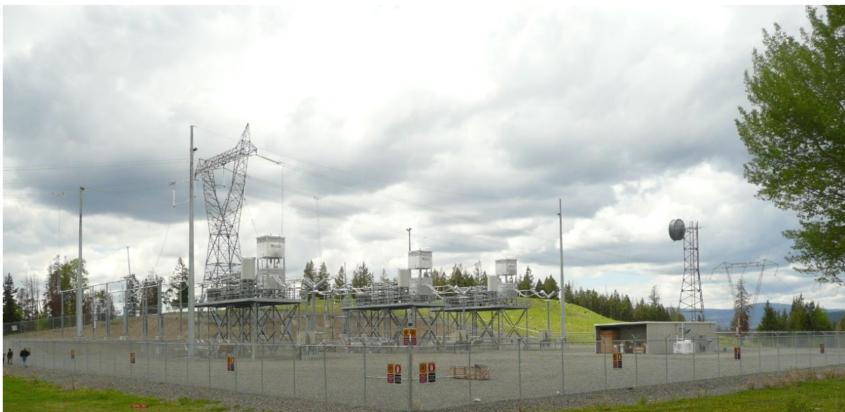
Photo 1: Typical capacitor station
