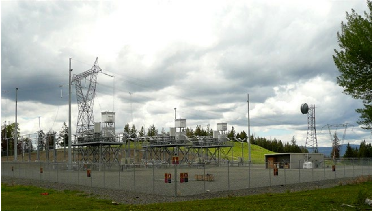
Figure 2. Example of a capacitor station - Guichon Capacitor Station near Logan Lake, B.C.
