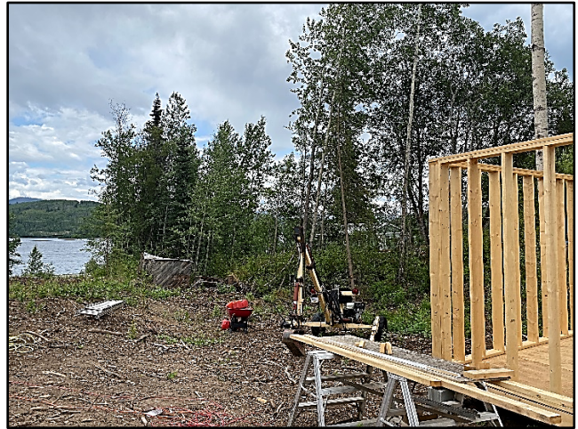
North view standing on proposed build site of east property slope and elevation changes
