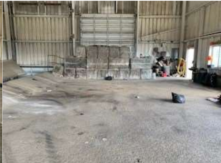
Figure 4 - Tip floor facing north. Note: Lock block wall at north end will be removed for resurfacing.
