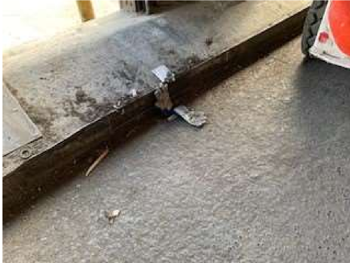
Figure 7 - Steel plate along public drop
