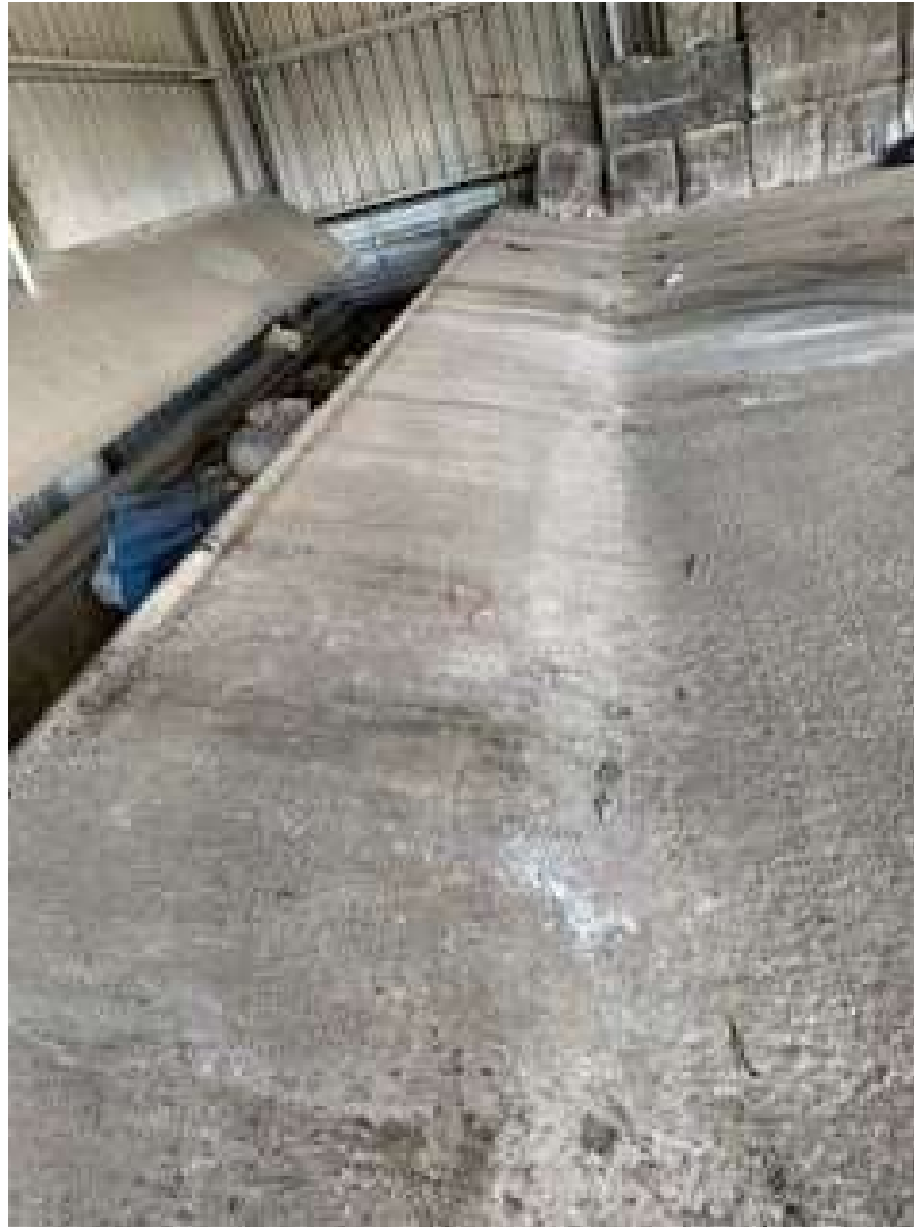
Figure 5 - Ramp facing north. Notice wear at transition
